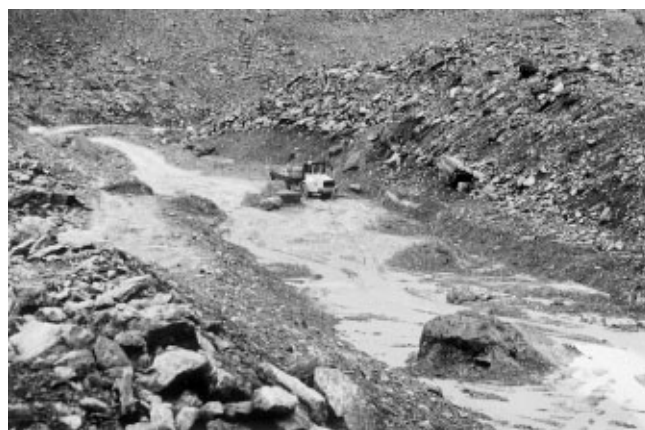
Fig. 13. Excavation of a drainage channel for ice-marginal Lake No. 3 (photo A. Kääb, 1995).
