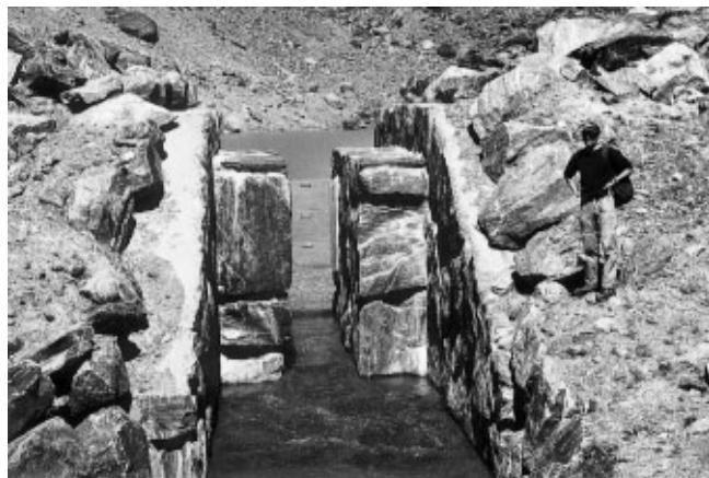
Fig. 14. New (lowered) flood-release (overflow) structure with regulating gates at proglacial Lake No. 1 (photo W. Haerberli, July 2000).
